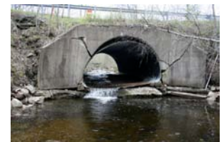
In 2010, this culvert on Shaker Mill Brook was replaced with a fish-friendly crossing.
