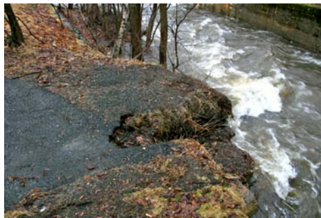
Paved drainage swale dumping road runoff into Yokum Brook in Becket
