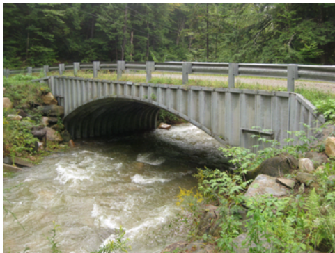
After previous floods washed out the road over Bronson Brook in Worthington, local partners replaced it with this bottomless arch culvert. Photo-monitoring documented that Tropical Storm Irene washed a large tree down to this crossing and the tree passed easily through this span.
